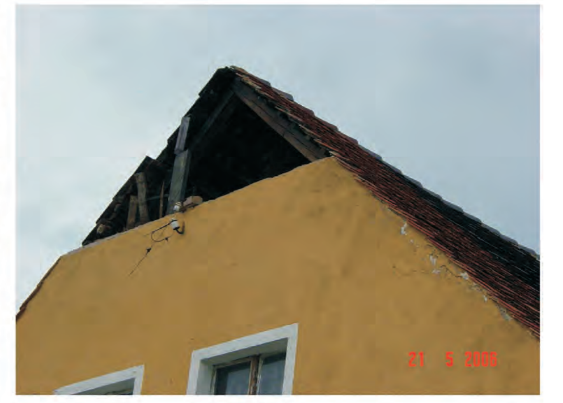
Fig. 3 Damage to a gable wall caused by mL 4.3 rockburst from May 21, 2006 in Polkowice, Poland.
